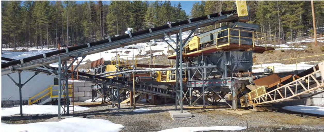
Figure 17.3 Conveyor, Cone Crusher and Vibrating Double Deck Screen
