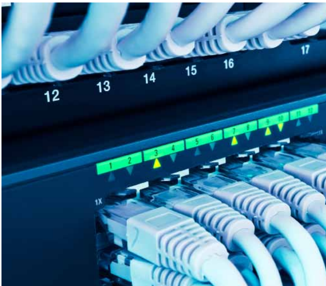
Telecommunication Infrastructure at Ras Al-Khair
