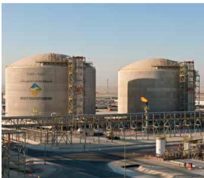
Storage tanks at Ras Al-Khair
