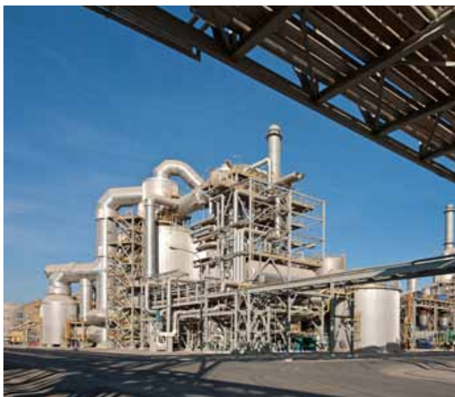
The sulphuric acid plant at Ras Al-Khair
