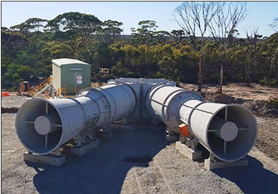
Figure 16-26: Typical surface fan installation
