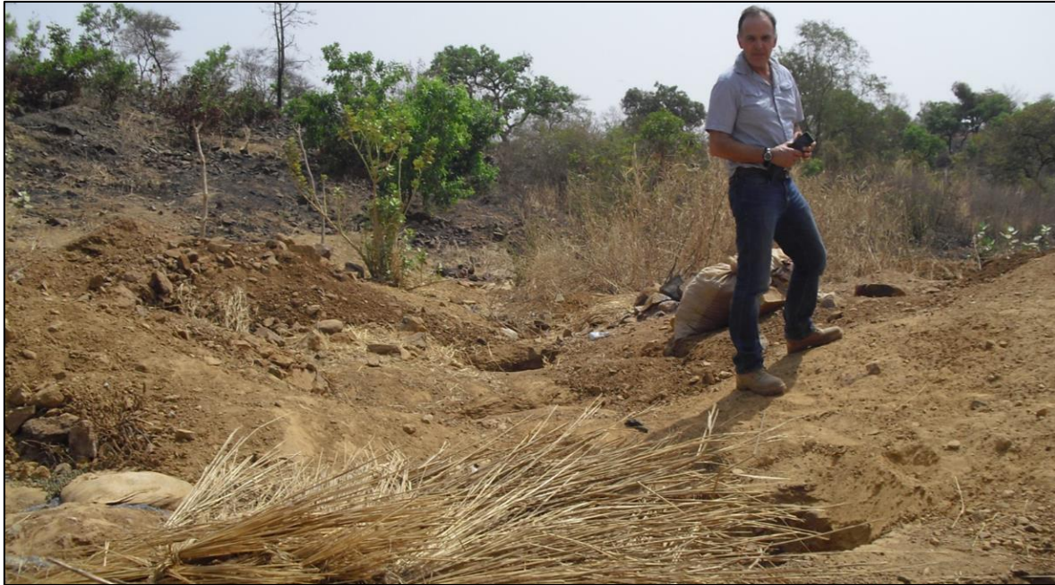
Figure 2-1: Artisanal mine shafts at Netiana, Balogo Project (Dr Matthew Randall looking on)
