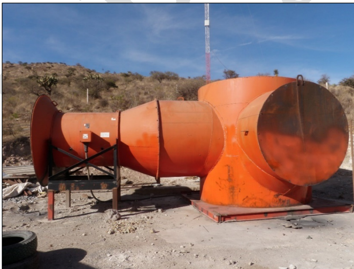
Figure 64: Quebradillas Exhaust Fan (SRK 2017)
