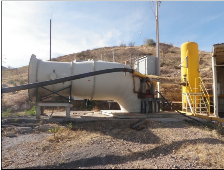
Figure 63: Intermedia Exhaust Fan (SRK 2017)
