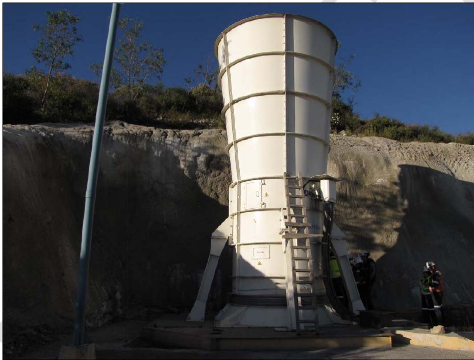
Figure 62: Rosarios Main Exhaust Fan (FSM 2017)
