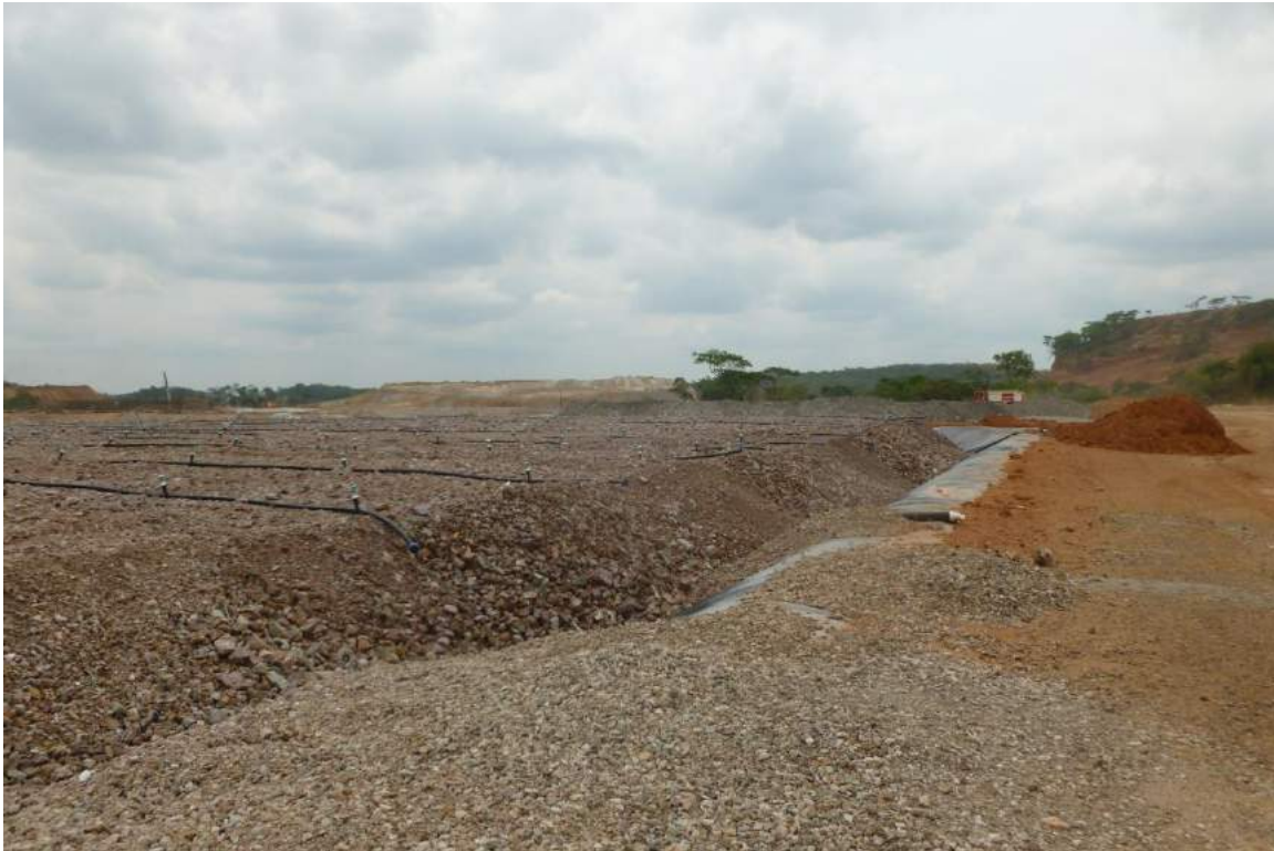
Figure 13-2 Heap Leach Pad
