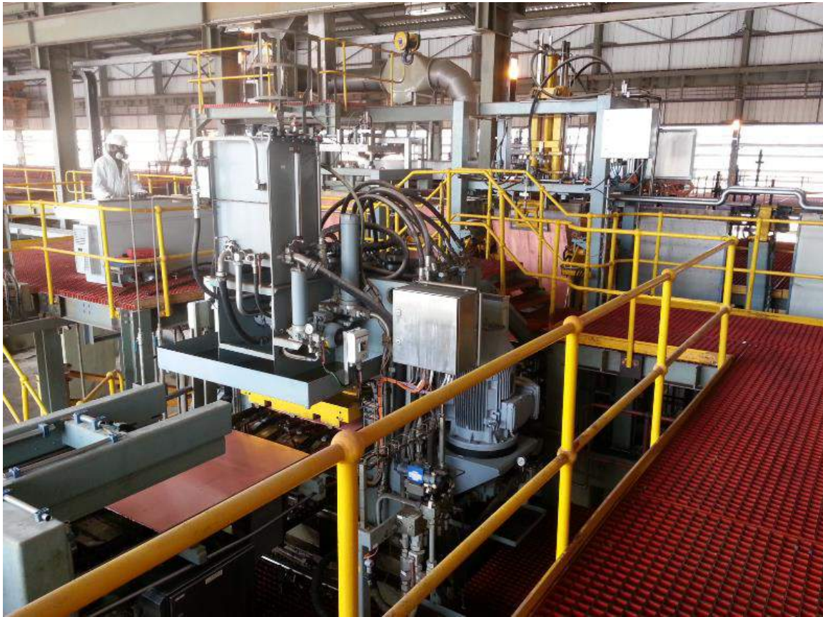
Figure 17-4 New Automated Stripping Machine (November 2013 Site Visit)
