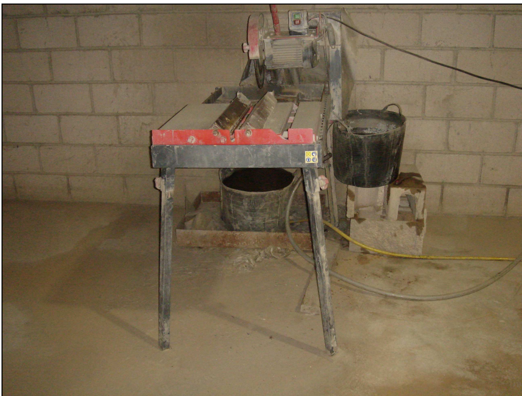
Figure 10-6. Core Sawing Facility
