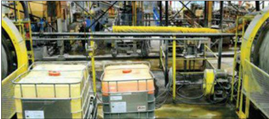
Installed Equipment in the Mill
