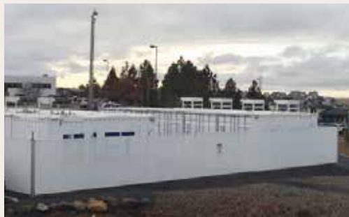
Operational 4MWh vanadium redox flow battery
