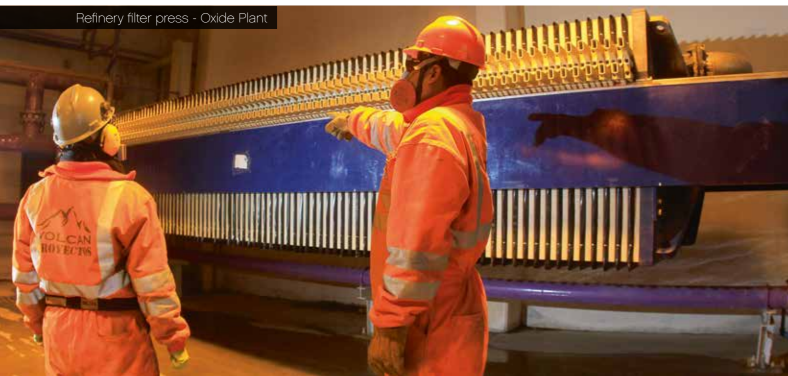
Merrill Crowe – Oxide Plant
