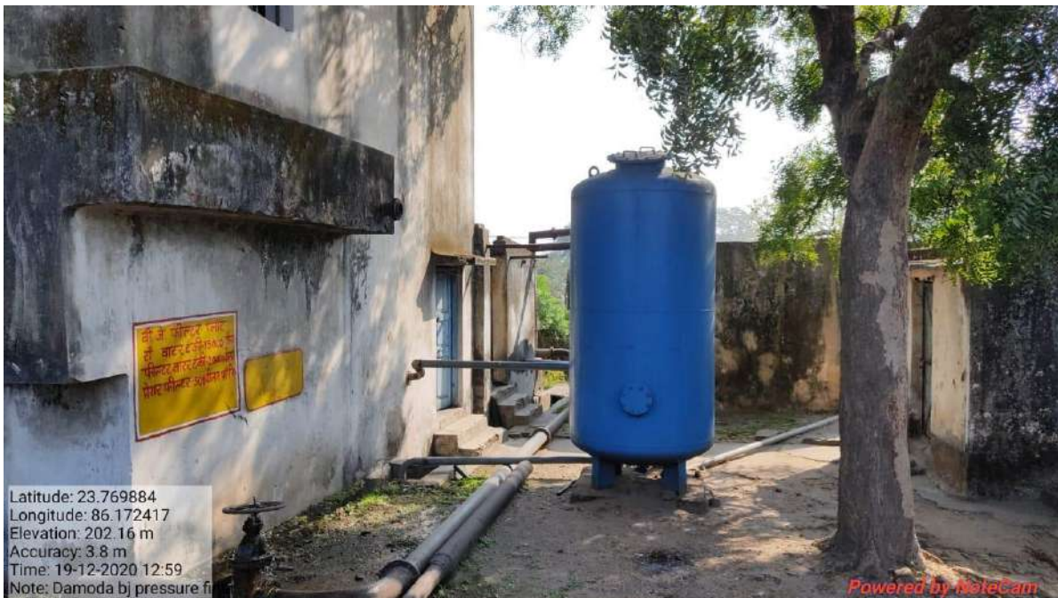
FILTER PLANT IN THE MINE AREA
