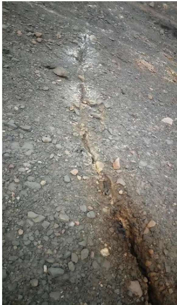
Figure 20: Fume cracks in the Bhulanbarari area.
