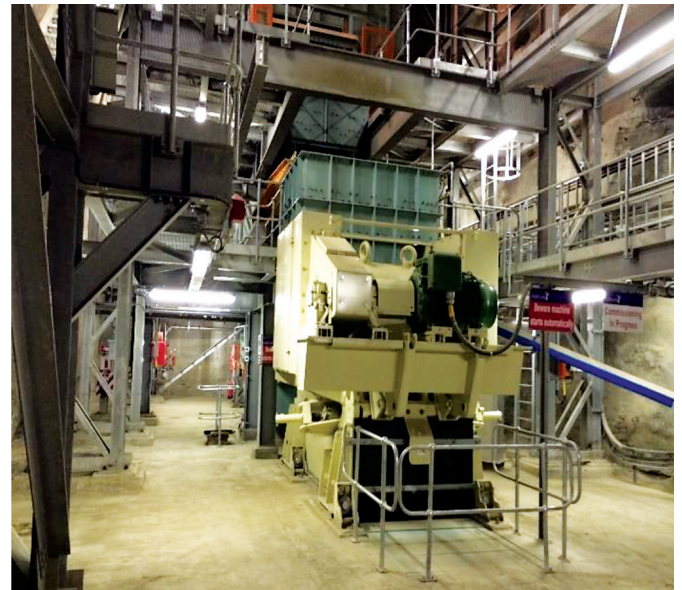
Figure 14. Portal 3 (Mupfuti Mine) underground crushing station
