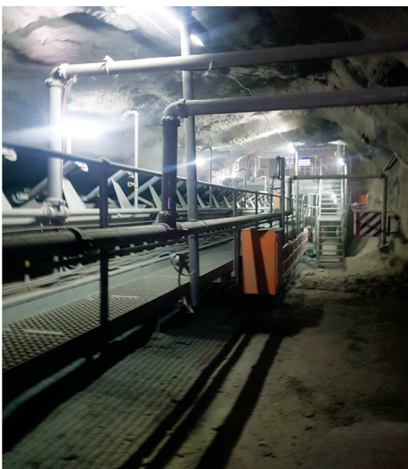
Figure 11. Portal 4 (Bimha Mine) sacrificial conveyor
