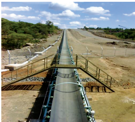
Figure 8. Portal 1 Overland conveyor
