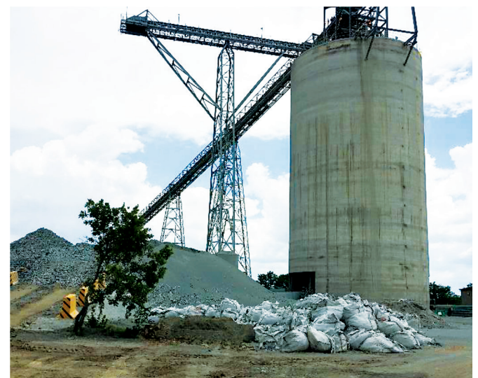
Figure 15. Portal 3 overland conveyor with silo by-pass
