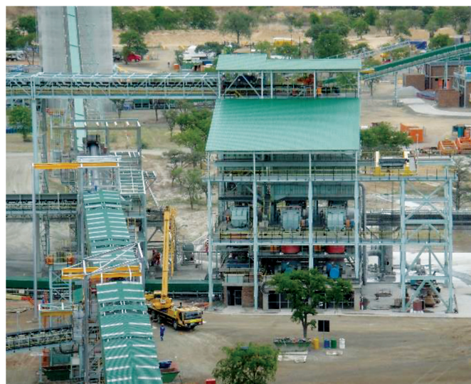
Figure 17. Ngezi Concentrator secondary crushing and screening
