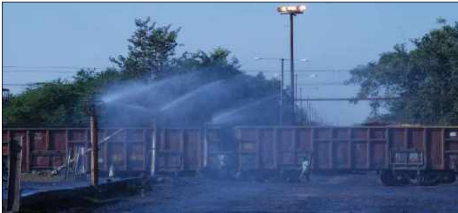
Fig 7: Fixed Sprinkler System at Railway Siding
