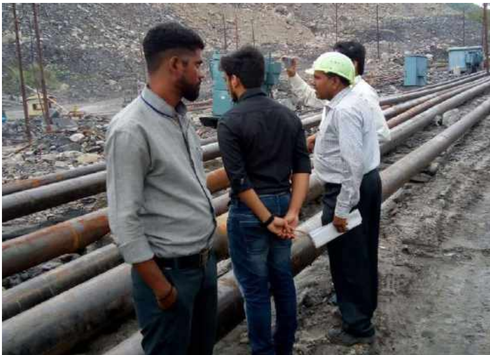
Fig.2.16. (A):- Water disposal system at the mine site.
