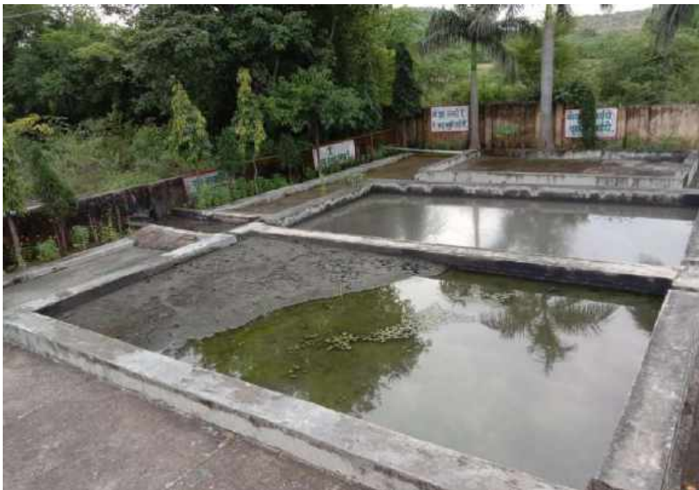
Fig.2.15.(B):- Effluent Treatment Plant for mine water.
