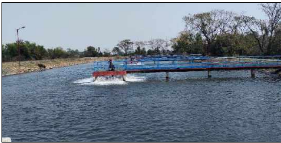
Fig 31: Domestic Effluent Treatment Plant (Combined with Gevra Project)
