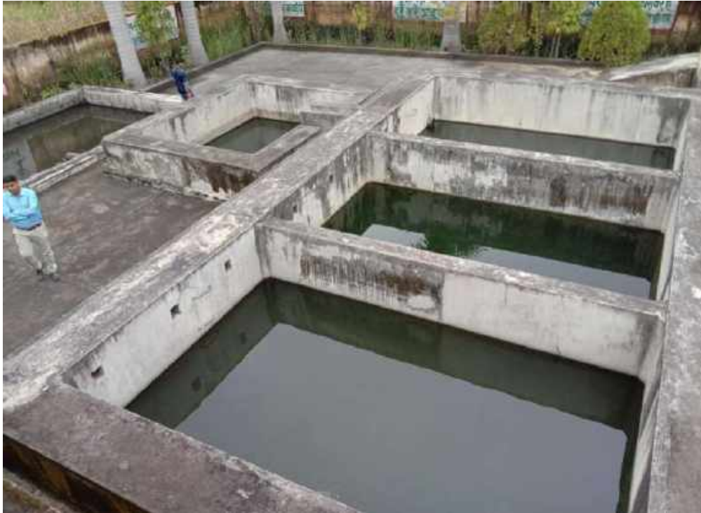
Fig.2.15.(C):- Effluent Treatment Plant for mine water treatment.
