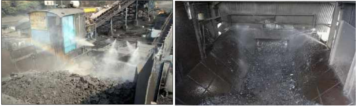
Fig 1: Feeder Breaker with Mist Spray Arrangement System
