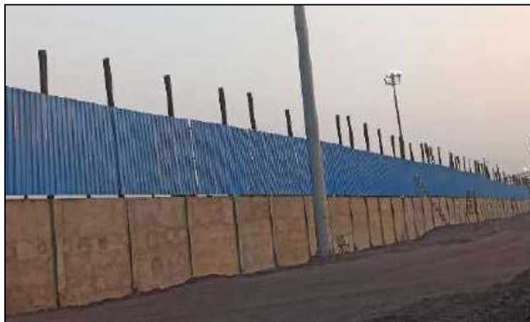
Fig 3: Construction of Wind Barrier Wall with Brick work and GI sheeting on both sides of Railway siding
