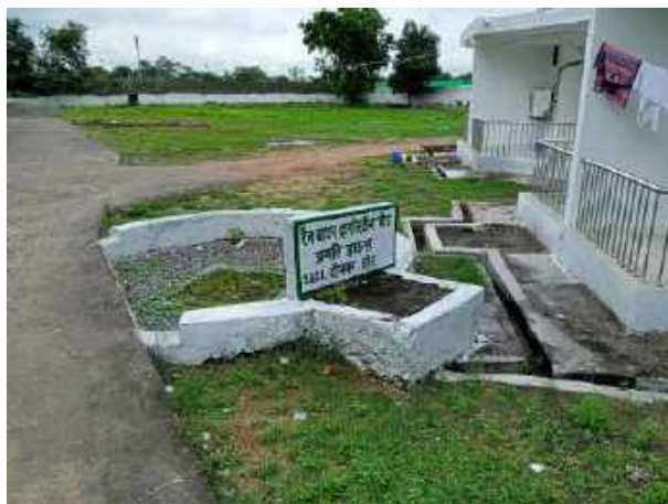
Plate 25: Rain water harvesting pit with open drain at Pragati house, Dipka OCP
