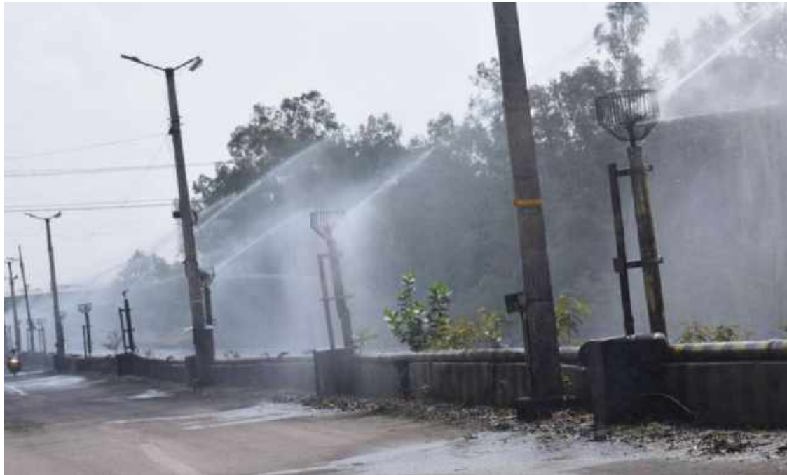
Fig. 2.11: Water sprinkling system along the road for control of dust during coal transportation
