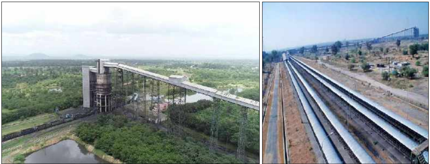
Fig 20: Inpit Belt Conveyor System
