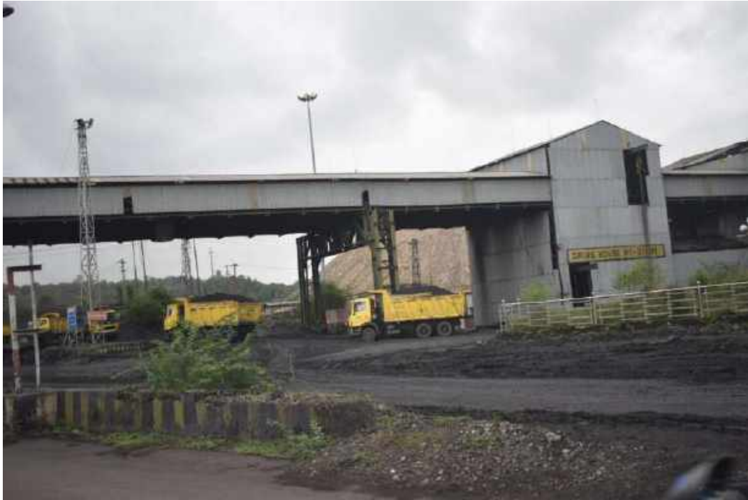
Fig. 2.12: Transportation of coal through a covered conveyor belt.
