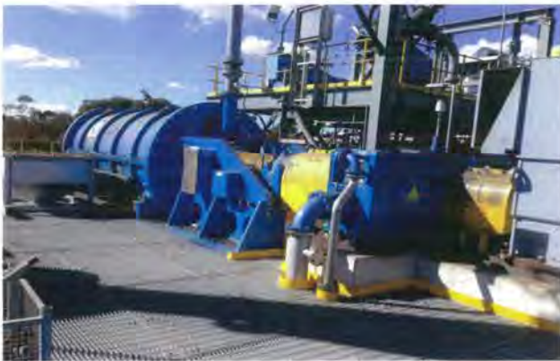
FIG 4 – Kalgoorlie Consolidated Gold Mines' M10 000 IsaMill™ installation.
