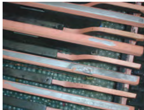
Figure 2: Corrosion of copper coating after 7 years operation
