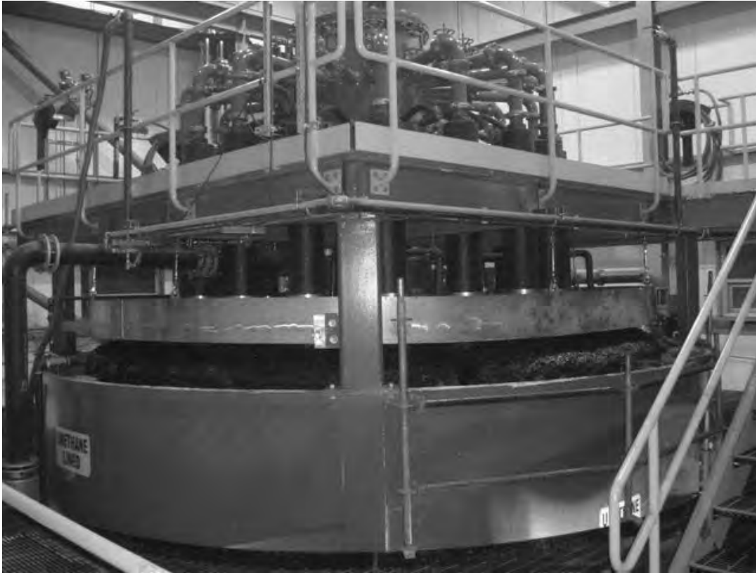
Figure 6: The preflotation Jameson Cell during commissioning at Red Dog Mine.
