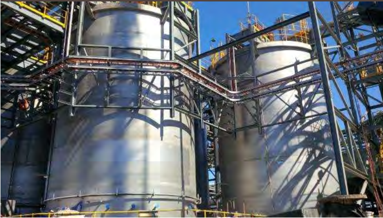
Oxidative Leach circuit
