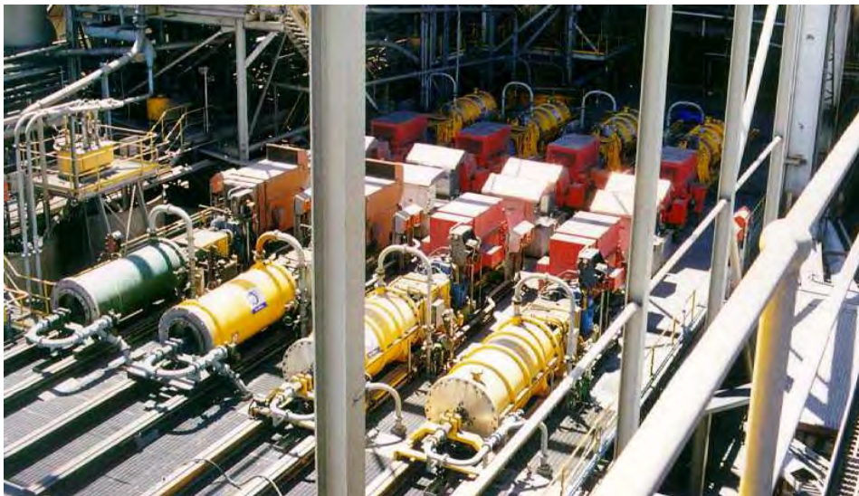
Figure 1: IsaMills in the Regrind Circuits at the Mount Isa Mines Lead/Zinc Concentrator
