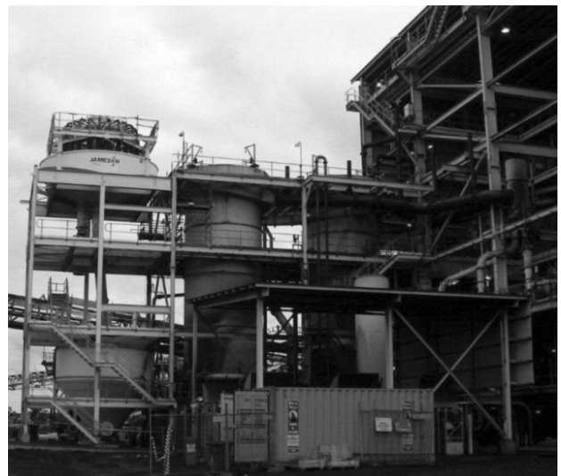
Figure 8: Recently installed Jameson Cell (left) next to two column cells at AAMC's German Creek operation
