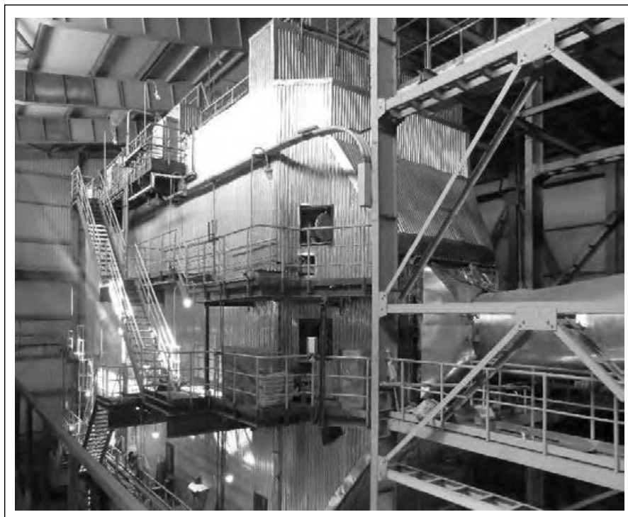
Figure 4: ESP in the Lead plant
