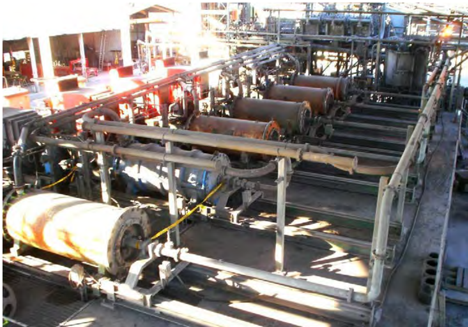
Figure 3 - 6 x M3000 IsaMills™ at McArthur River
