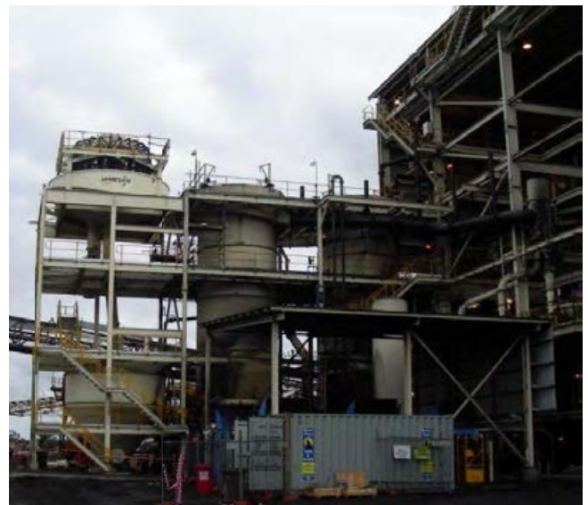
Figure 8: Recently installed Jameson Cell (left) next to two column cells at AAMC's German Creek operation
