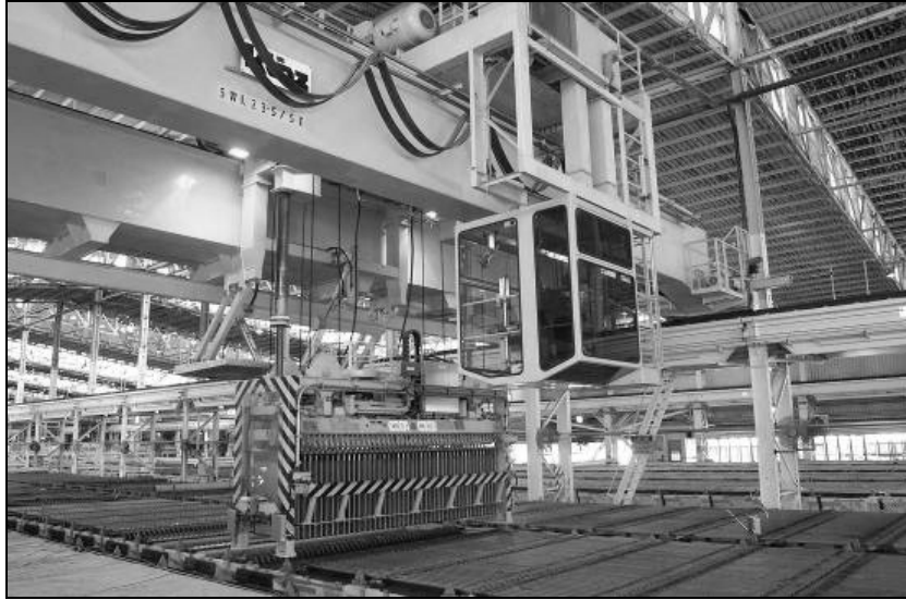
Figure 8 – Tankhouse Overhead Crane
