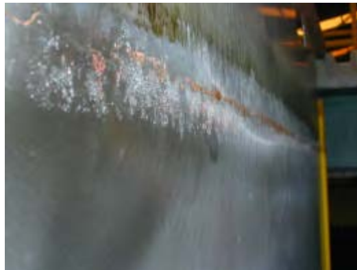
Figure 4: Solution line corrosion
