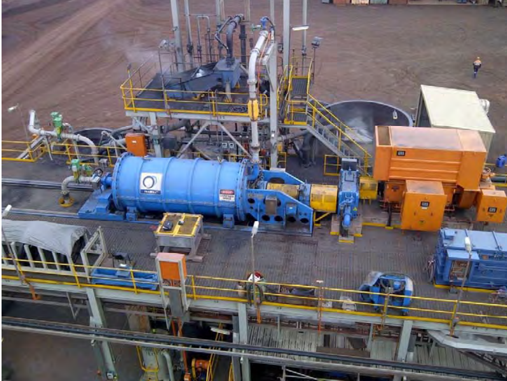
Figure 6 – Arrium M10000 IsaMill installation.
