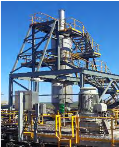
Off Gas Scrubber
