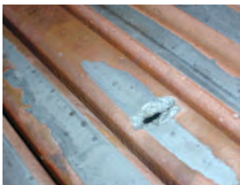
Figure 5 Damage caused to hanger bar from incorrect use of shorting frame
