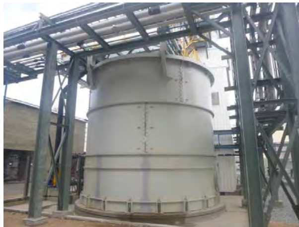
Figure 5 – Limestone storage tank.
