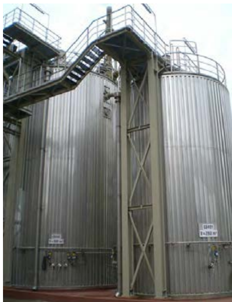
Figure 6 Albion Leach Reactor at Nordenhams
