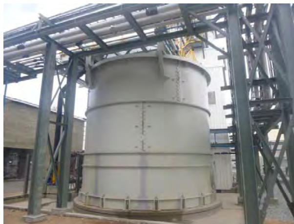
Figure 5 – Limestone storage tank.
