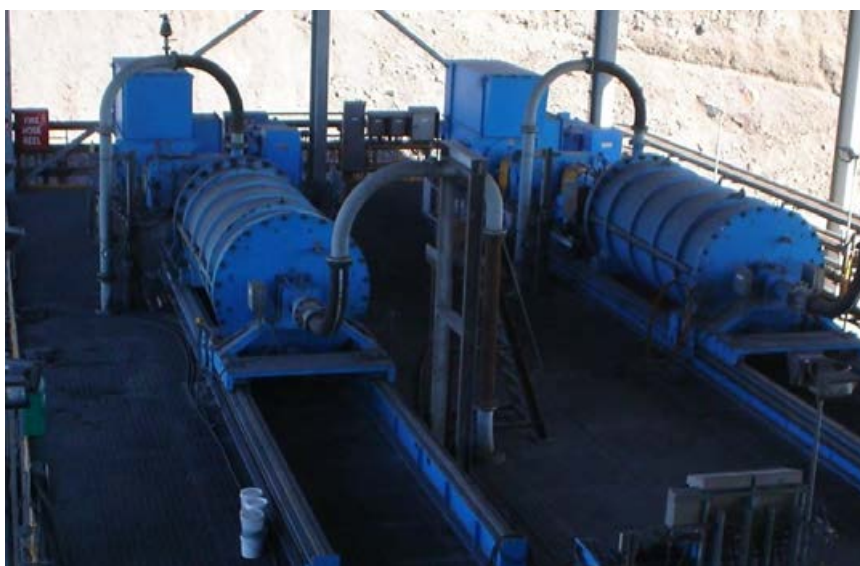
Figure 11 - 3.0 MW M10,000 IsaMills™ at McArthur River
