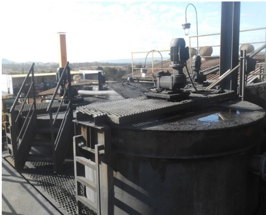
Figure 97 - CIL (Carbon-in-leach) Unit overview
