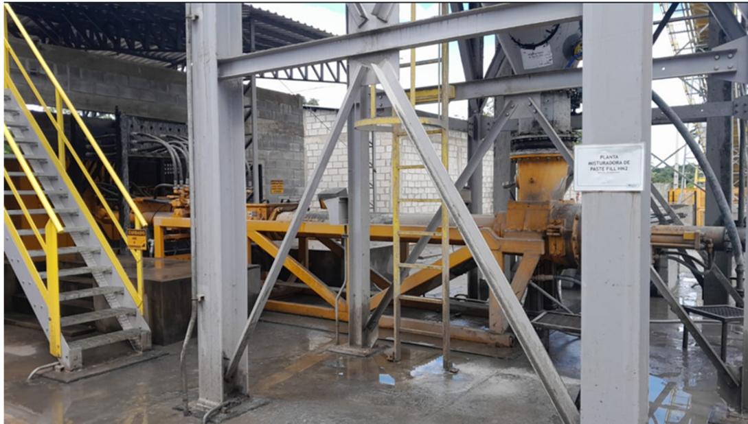
Figure 85 - Xavantina paste fill plant, Piston Pump Duplex KSP 220XL + EHS 4500 (Xavantina, 2022)
