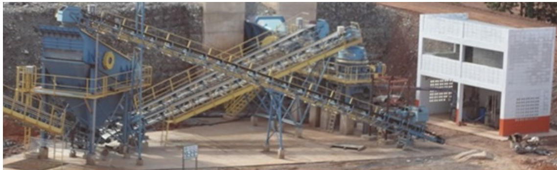
Figure 92 - Crushing Unit overview
