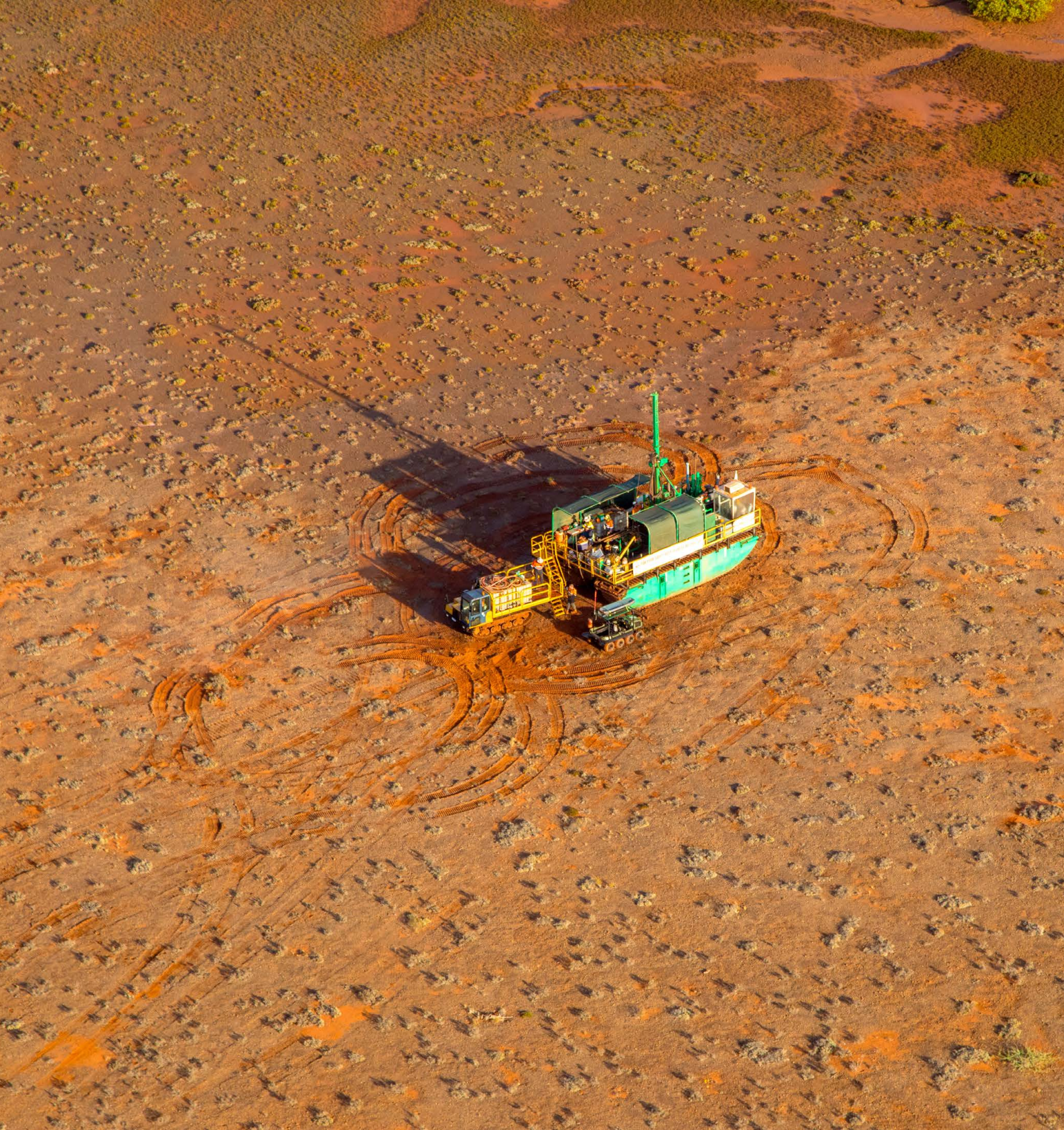
Geotechnical drilling within the evaporation pond footprint at the Mardie Salt & Potash Project
