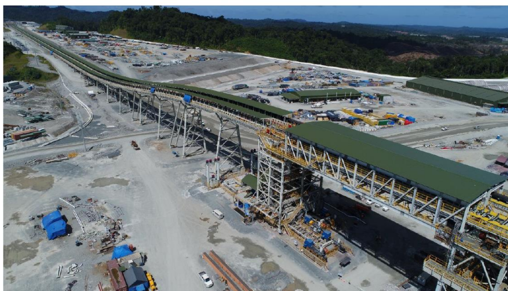
Figure 18-5 View of overland conveyors
