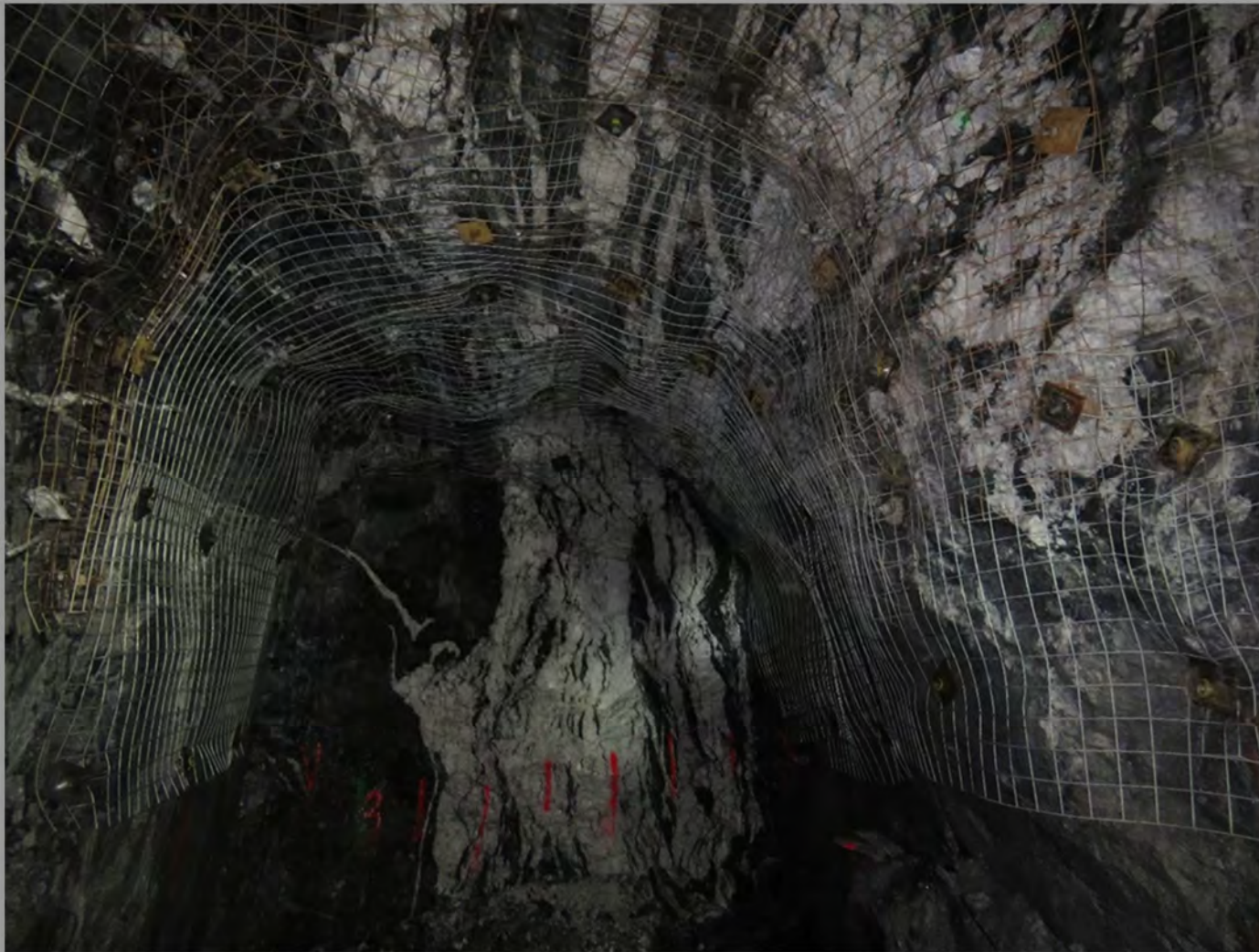
Figure 9.9 Level 3 West Round 30 - Steeply Dipping Breccia Quartz Veins Hosted in Argillite in Belt 2 (looking west)
