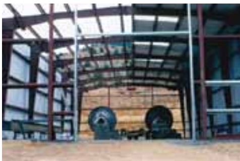
The Contact Mining Company Mill, located about a mile south of Philipsburg in part of the site of the old Bimetallic Mill. There are two big smokestacks just above the mill that went with the old Bimetallic Mill.
