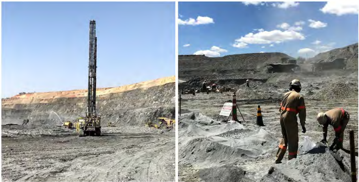
Figure 14-35: Blast hole drill rig (Pit Viper) left side and geology sampling team collecting samples on the drilled cones on the right side.
