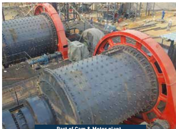
Part of Cam & Motor plant
