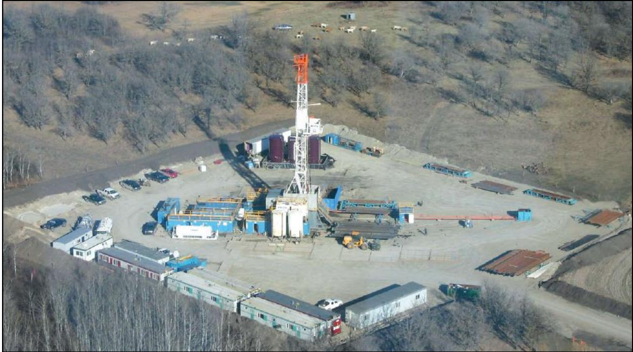
Figure 15: Drilling of pilot hole at the Scissors Creek shaft site in April 2009 (photo by K. Weedmark, Moosomin World Spectator).
