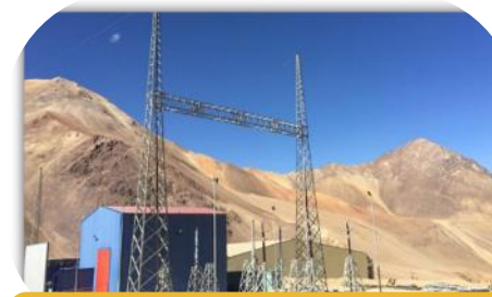
POWER LINE i
