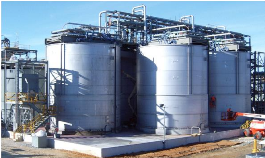
Figure 1.1 : Kirkland Lake Gold Fosterville (211 tpd) BIOX ® Plant, Australia
