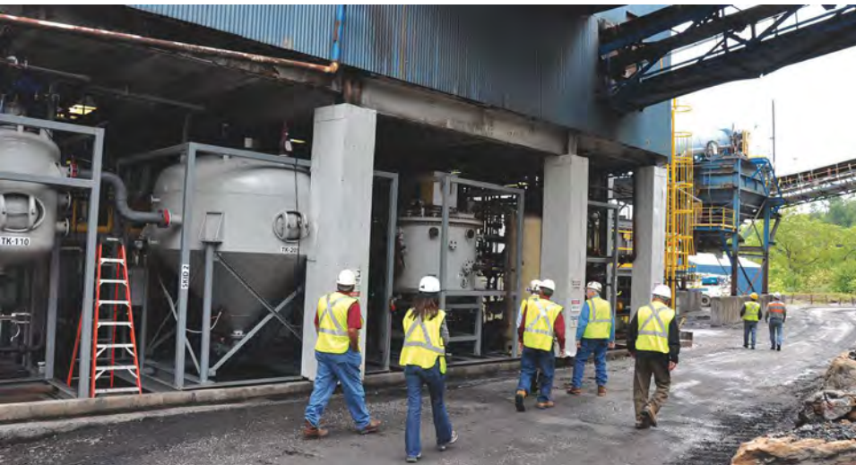
A group touring MRC's first commercial HHS plant strolls past the low-shear mixer, left, the phase separator, middle, and the Morganizer, right. (Photo: Minerals Refining Co.)
