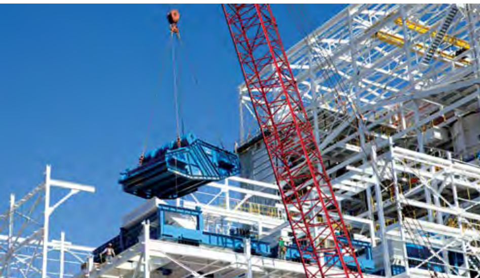
A Conn-Weld multislope screen is lowered into a new prep plant under construction.
