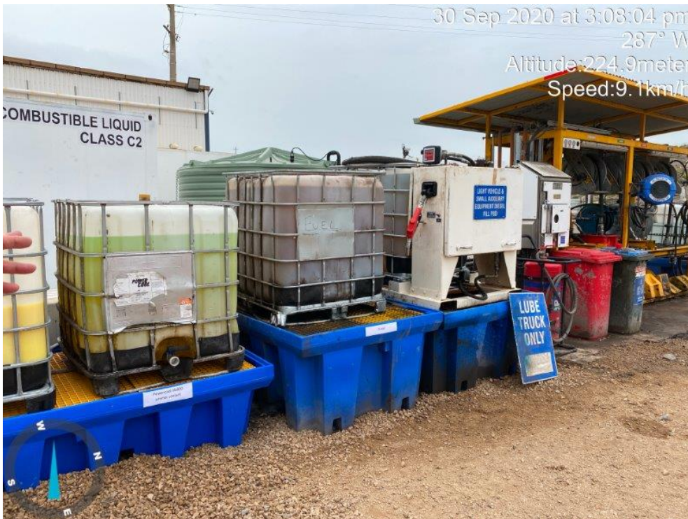
Photo 11: Correct storage of hydrocarbons at the pit top (near workshop area)
