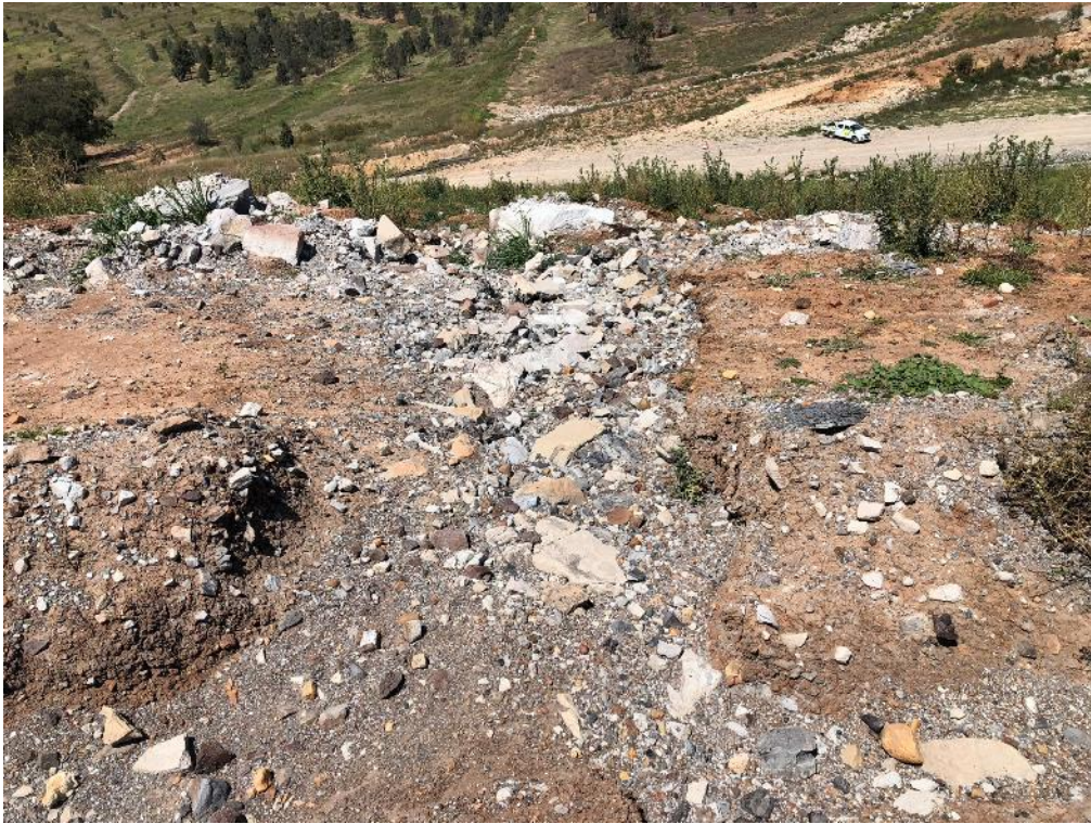
Photo 15: VD5 Gully erosion from dump crest bund failure – repair bund and reshape crest.
