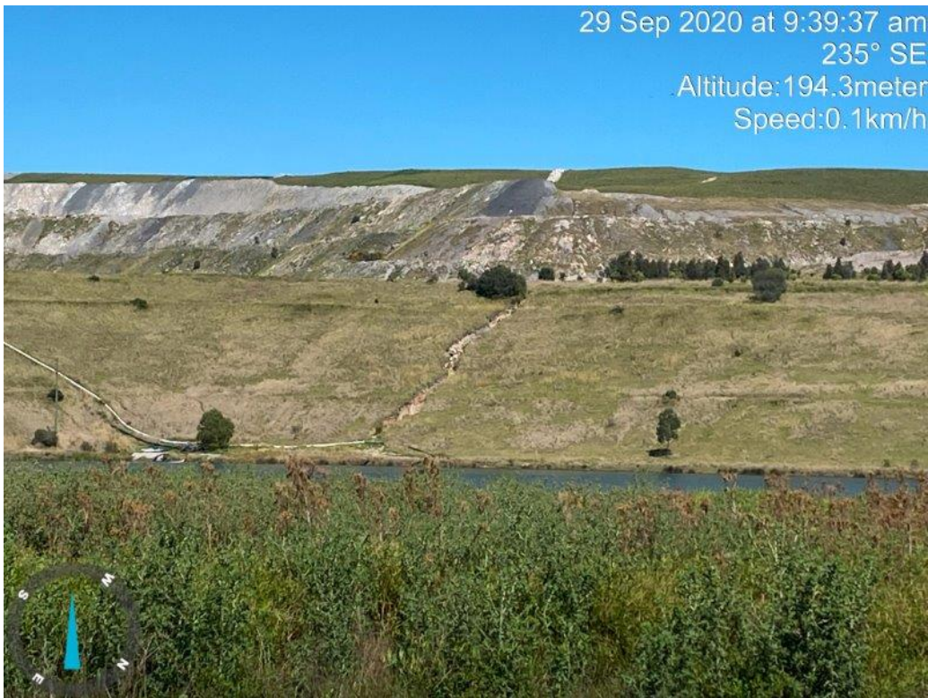
Photo 1: Erosion in Visual Bund. It is noted this area has plans for reworking.
