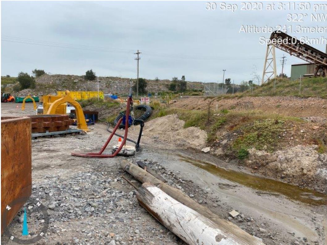
Photo 16: Minor water leak of a pipeline at the Thiess operational area. This is being contained onsite
