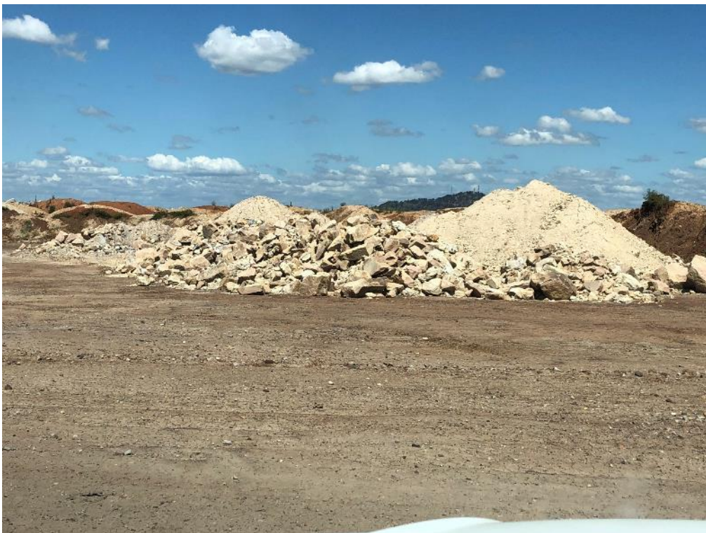
Photo 20: VD1 Competent rock being stockpiled for use in drainage lines on geomorphic landform designs.
