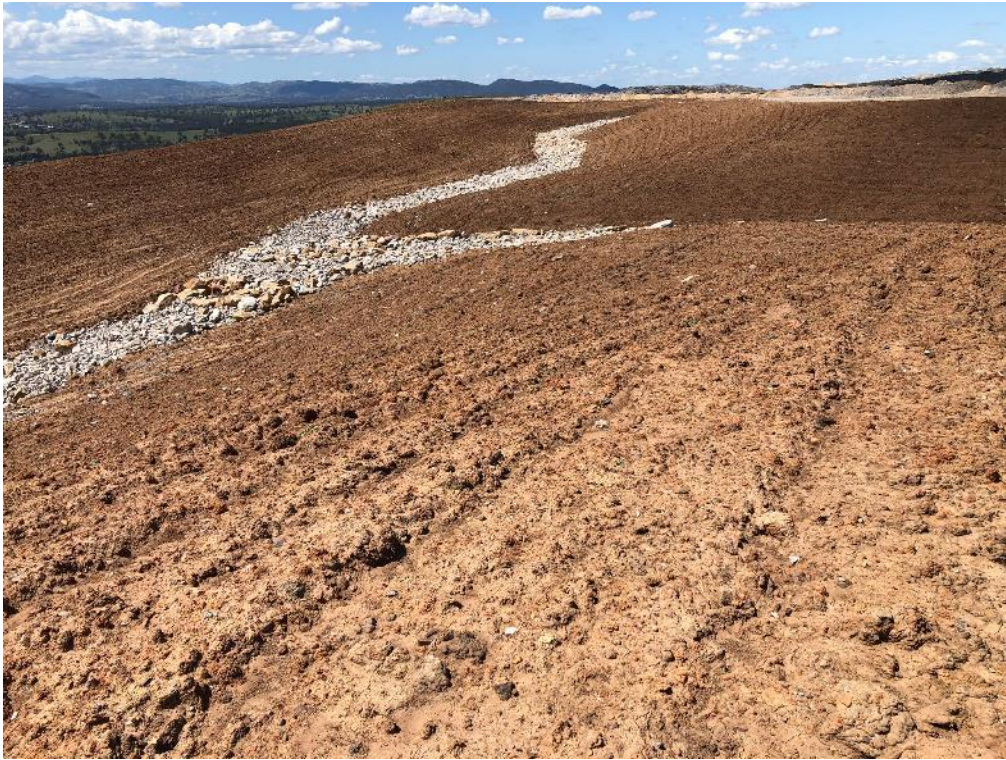
Photo 19: VD1 Geomorphic landform design being applied on site with rock lined drainage paths.
