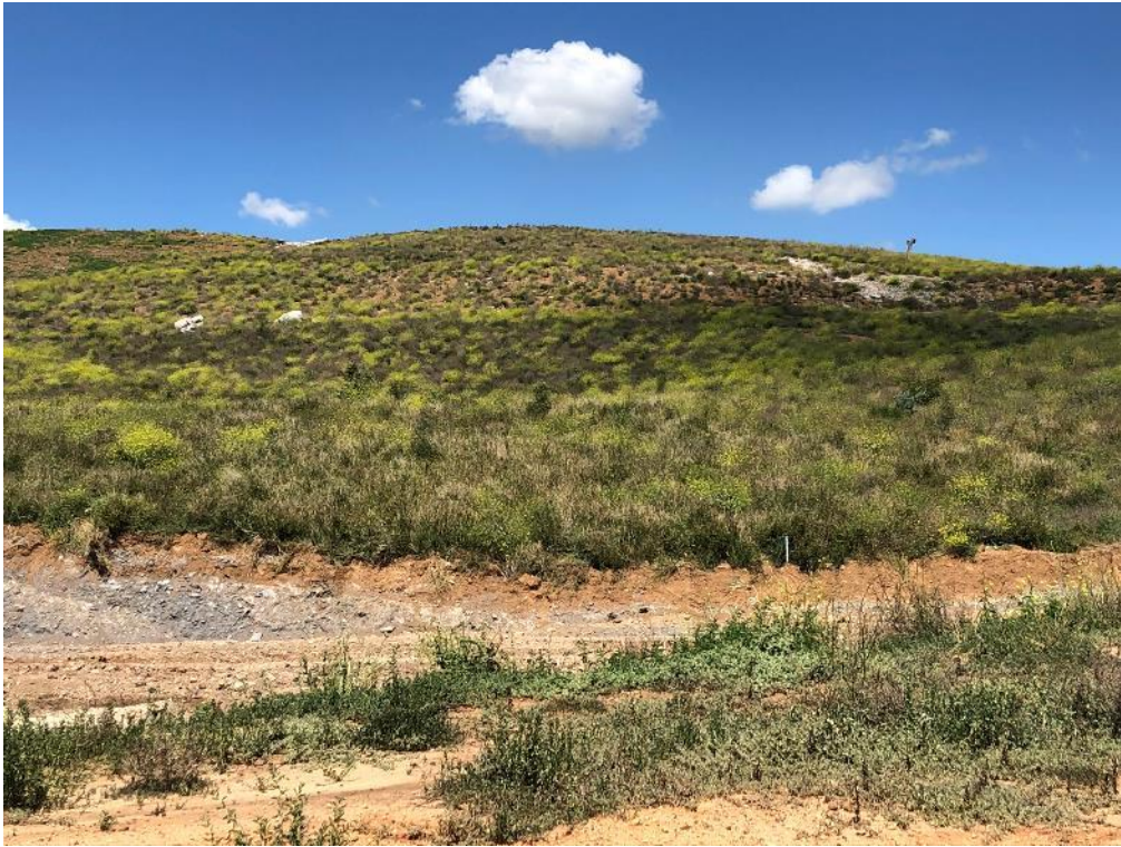
Photo 13: VD5 Soil surface and rehabilitation failure – implement planned re-rip and sow.
