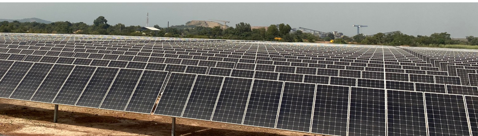
The Loulo-Goukoto mine complex has commissioned a 20MW solar power plant, with plans to double its capacity.
