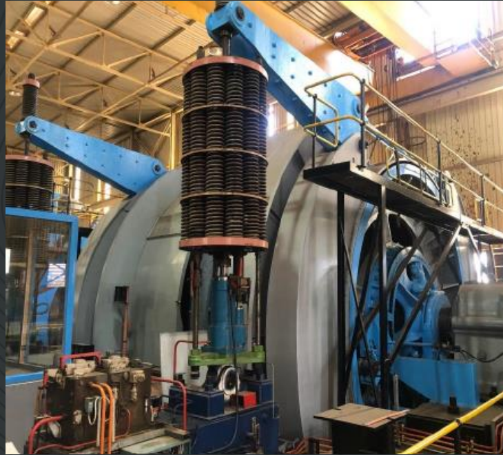
NO.5 SHAFT ROCK WINDER
