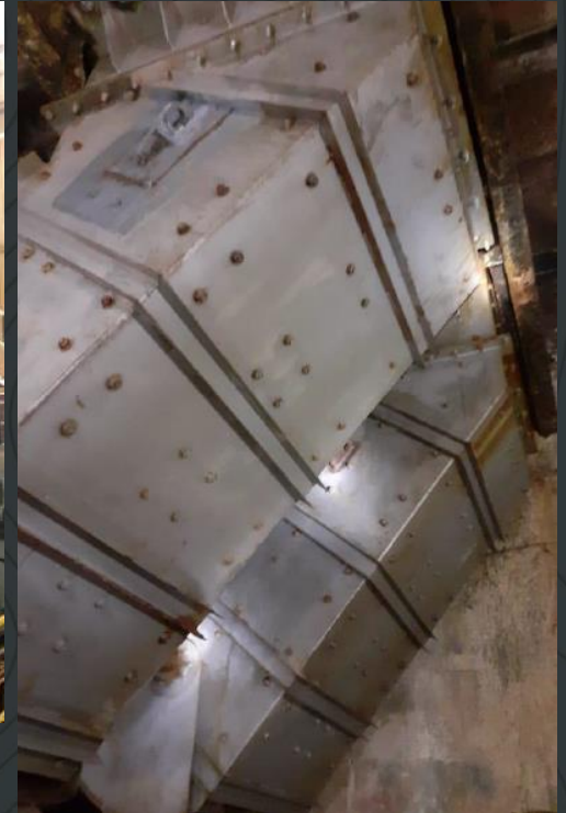
SHAFT LOADING BOXES LVL17
