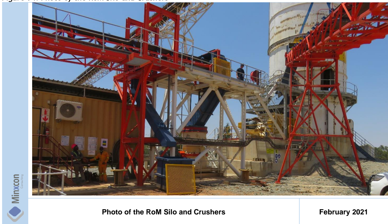
Figure 94: Photo of the RoM Silo and Crushers
