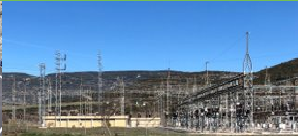
National Electricity Grid Substation is in close proximity to mine site
