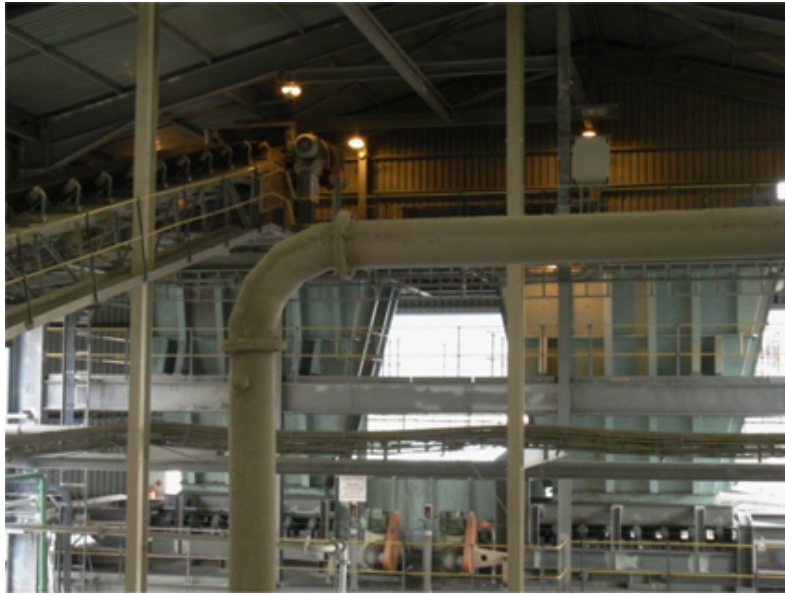
Figure 16.16: Merensky and UG2 filtered concentrate storage facilities.
