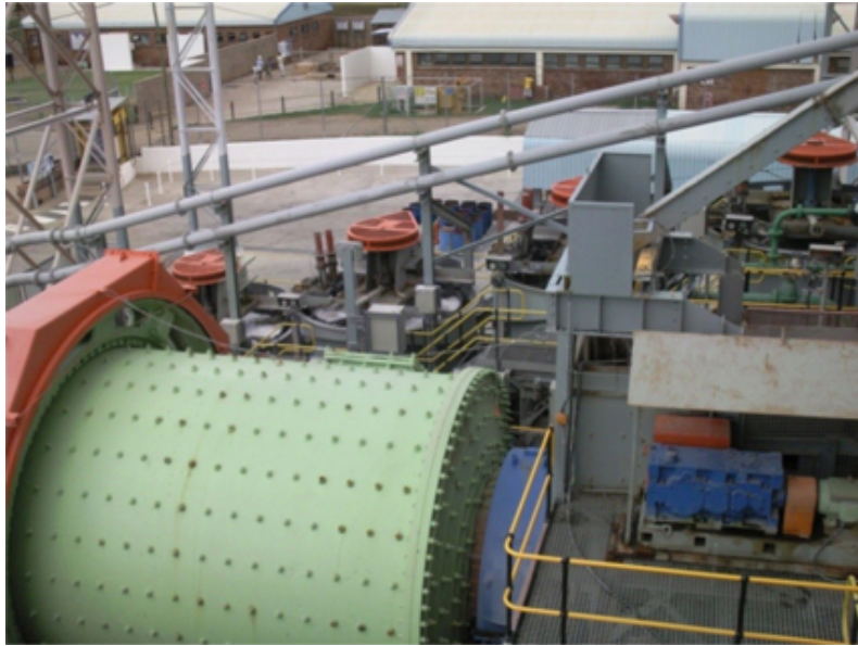
Figure 16.5: Primary FAG mill with the primary rougher smart cells in the background.
