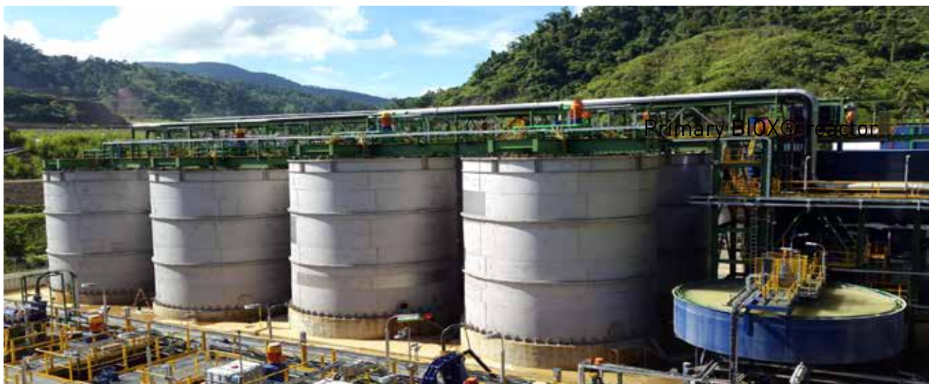
First implementation of the Generation III BIOX® circuit designed to treat 140,000 tpa of concentrate
