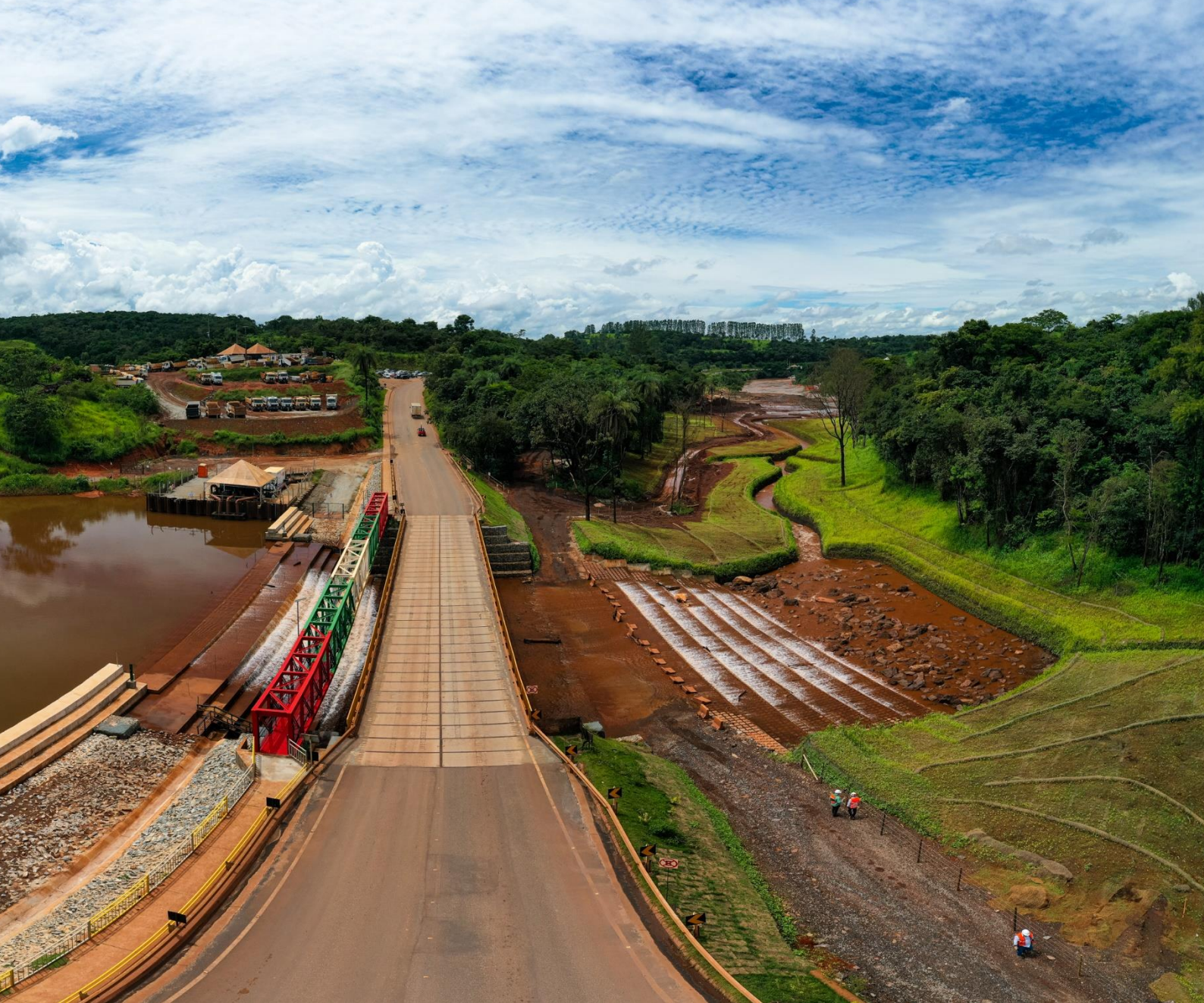
Zero Ground Project for environmental recovery in Brumadinho (MG) – section of the Ferro-Carvão stream
