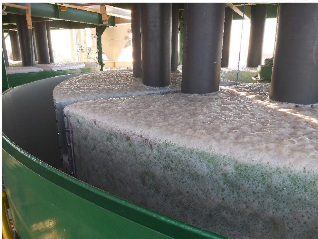
Figure 3: Process Plant flotation cell during commissioning
