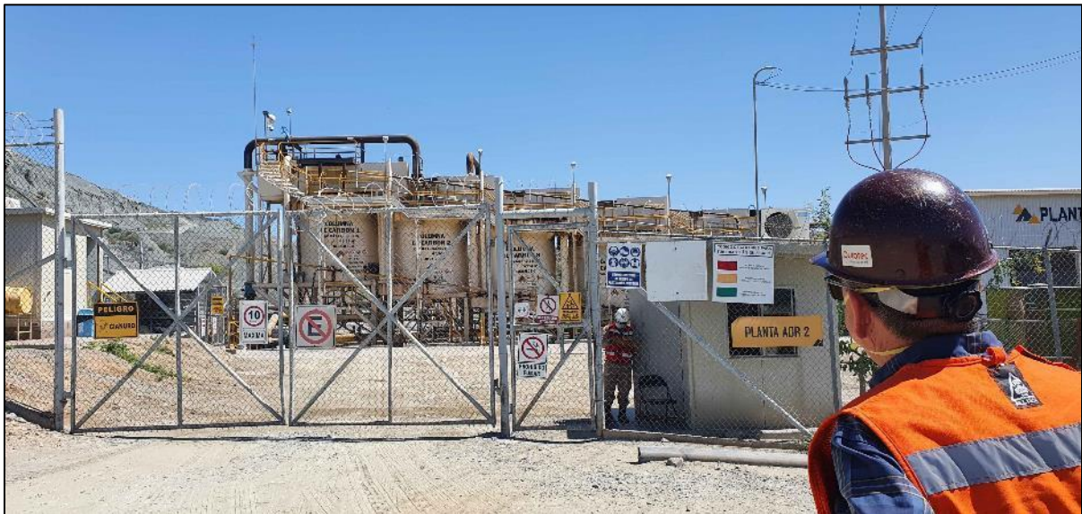
Figure 12.5 View of ADR Plant 2
