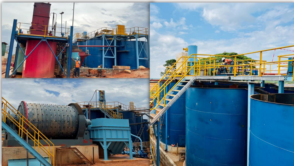
Buckreef Gold Expanded 360 TPD Processing Plant Integrated With 120 TPD Processing Plant
