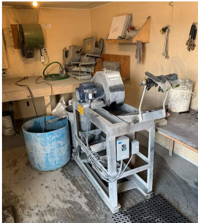
Figure 12-7: The Company core cutting facility
