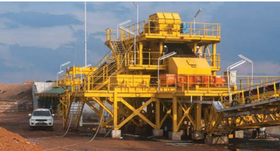
This crushing station, engineered by Metso Outotec and Komatsu, which includes a truck dump hopper, feeder and sizer (orange), is installed at PT Titan Infra Energy's Muara Lematang mine in South Sumatra.
