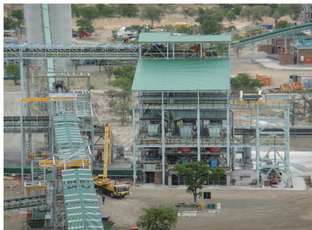
Figure 18. Ngezi Concentrator secondary crushing and screening
