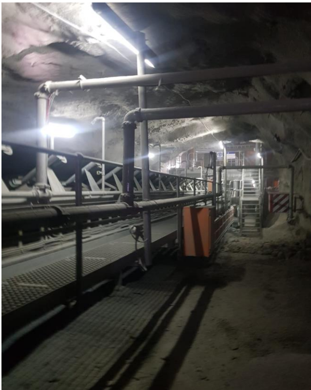
Figure 12. Portal 4 (Bimha Mine) sacrificial conveyor
