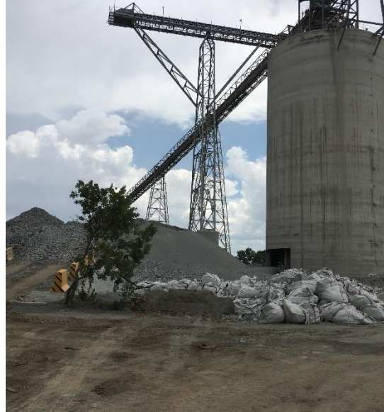
Figure 16. Portal 3 (Mupfuti Mine) overland conveyor with silo by-pass
