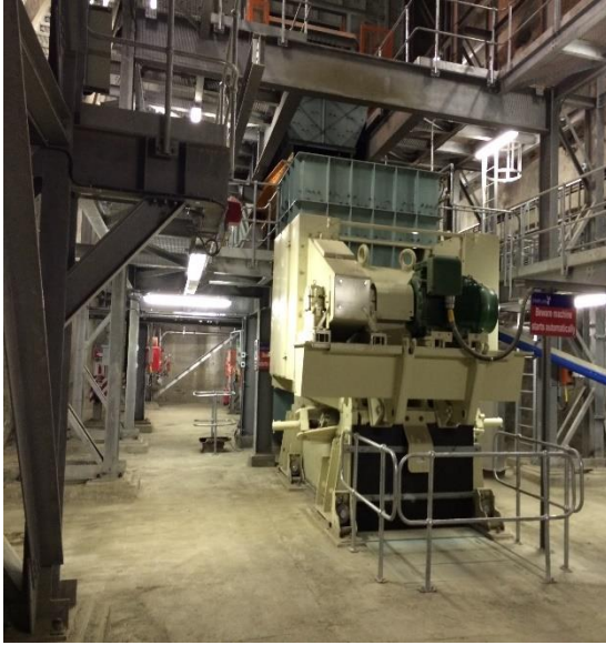
Figure 15. Portal 3 (Mupfuti Mine) underground crushing station
