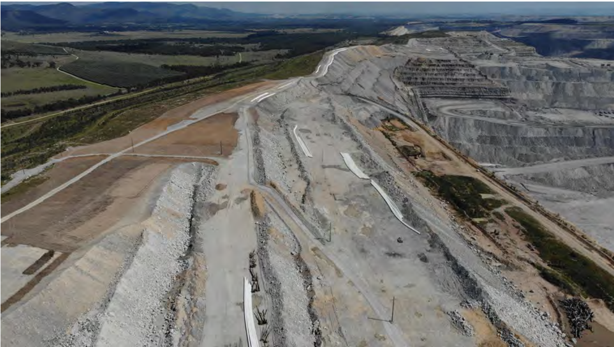
Photo 8 The natural landform design was integrated with the existing landform and drainage on the NVB, photo showing topsoil application in progress following shaping of the final landform.
