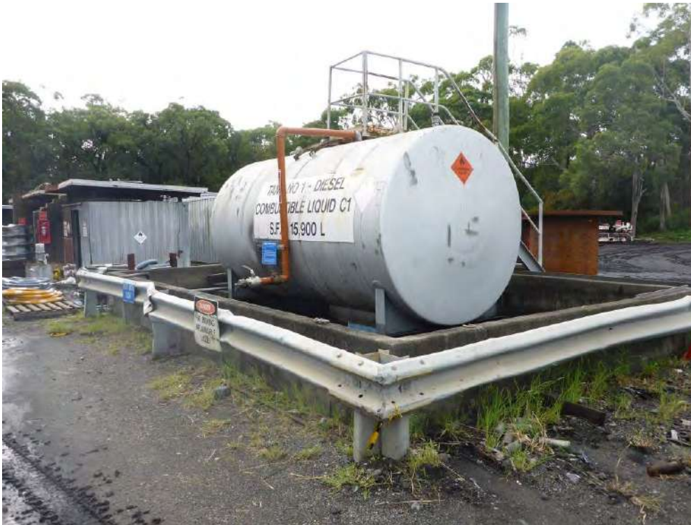
Photo 5 Diesel Tank stored within Bund
