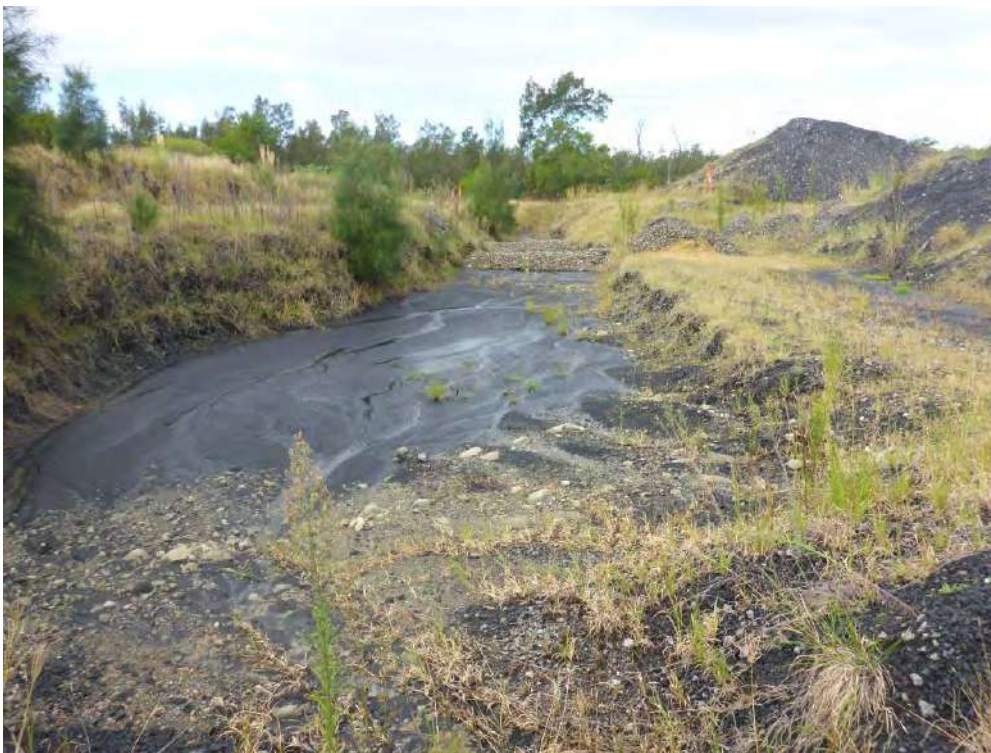
Photo 6 Coal Material in drain should be removed
