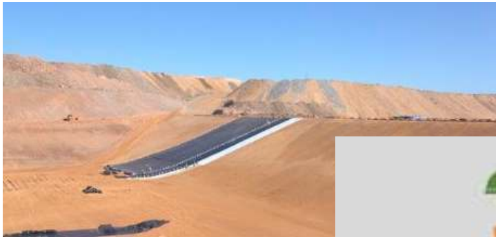
Geosynthetic to prevent seepage from a Tailings Storage Facility (TSF) at “La Herradura”
