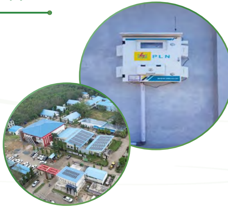
Figure 24: Installation of electric generator at Bunati Port (right) and solar panels on the offices' rooftops (left)
