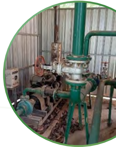
Figure 31: Neutramill machine installed at BIB's site
