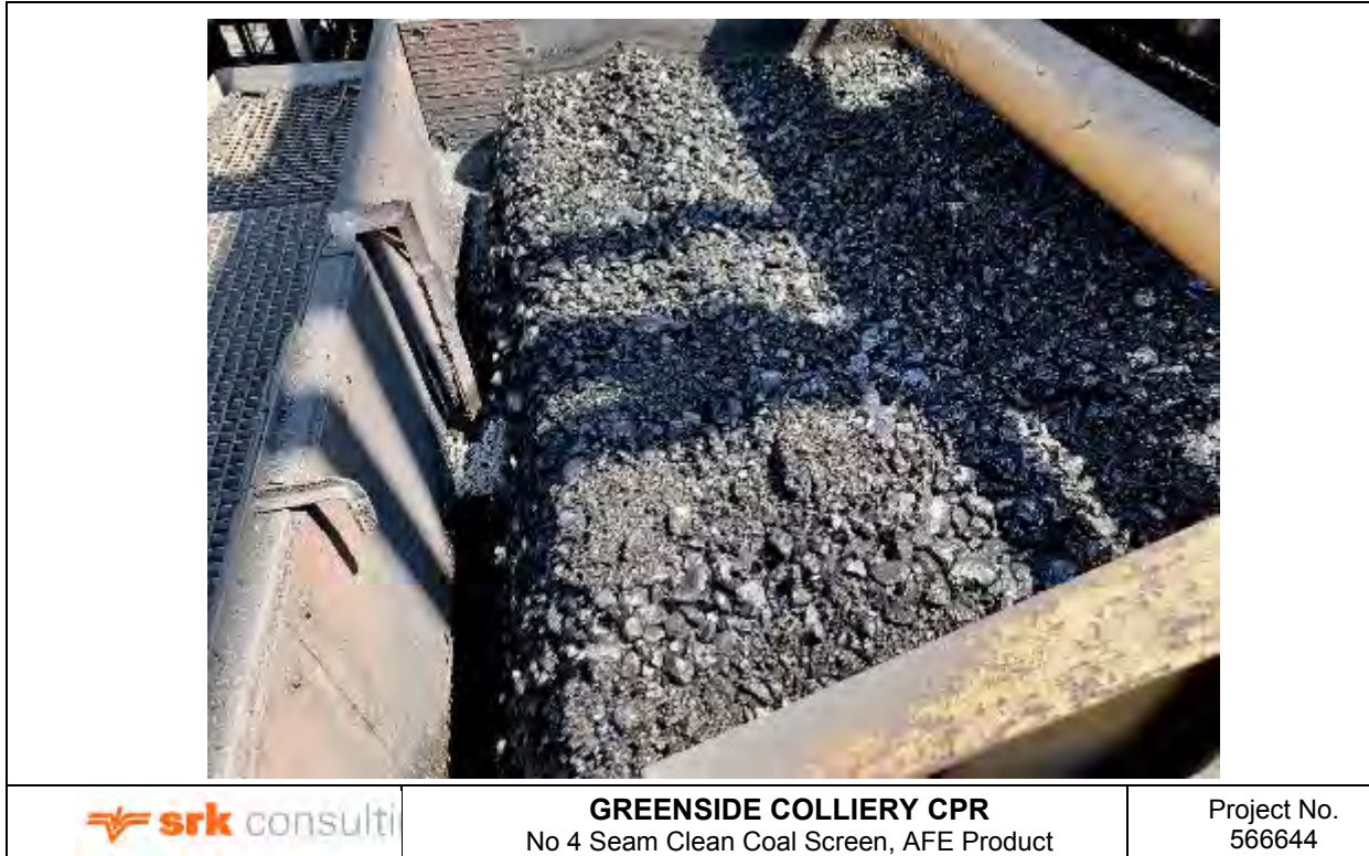
Figure 10-11: No 4 Seam Plant Clean Coal Screen
