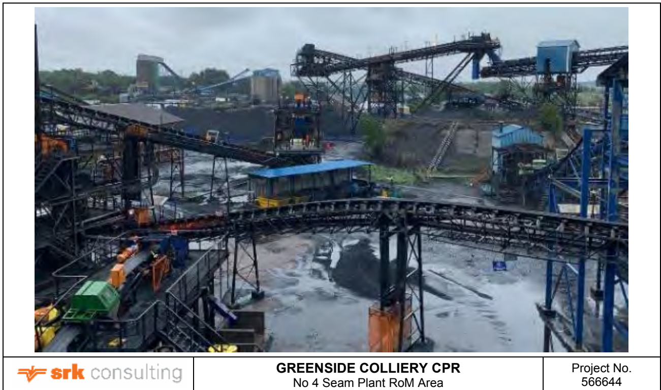
Figure 10-4: No 4 Seam Plant RoM Area
