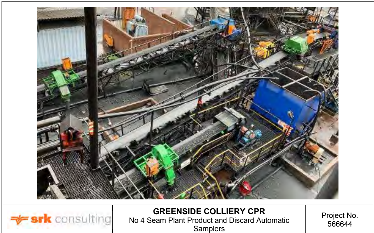
Figure 10-35: No 4 Seam Plant Product and Discard Automatic Samplers
