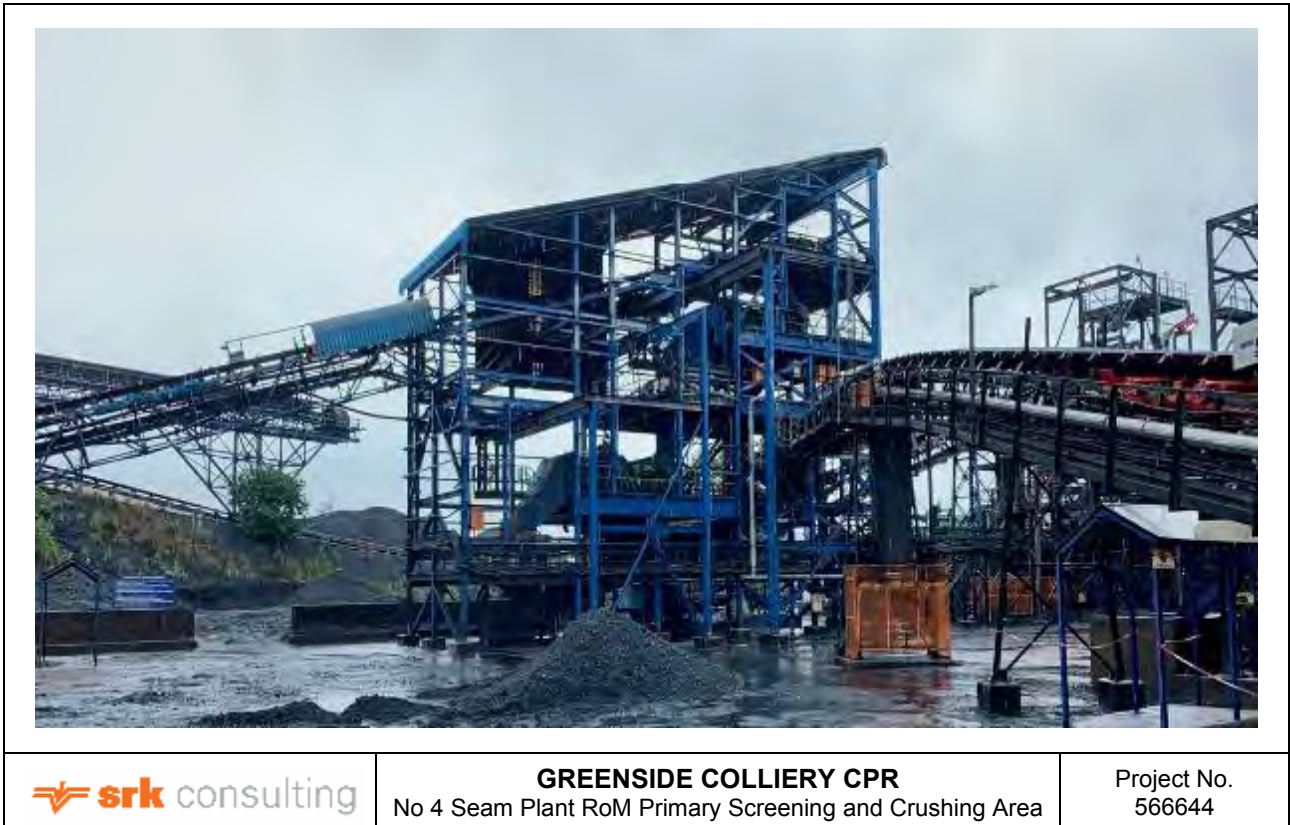
Figure 10-7: No 4 Seam Plant RoM Primary Screening and Crushing Area
