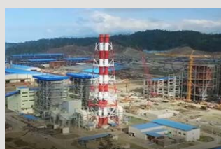
1.2GW power station &amp; coal plant
