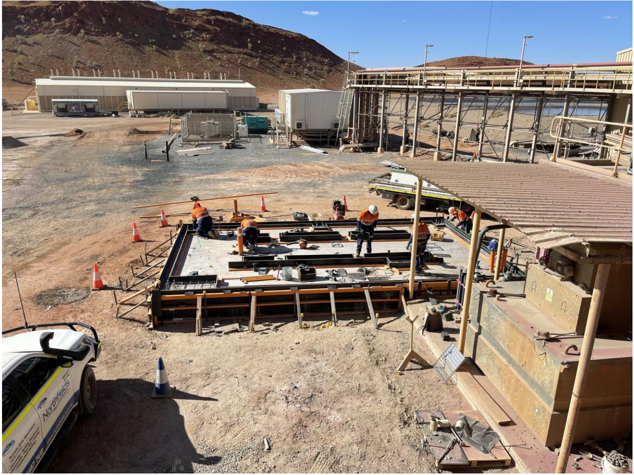
(Figure 5: Foundation works being completed for the new Acacia reactor unit – view facing west.)
