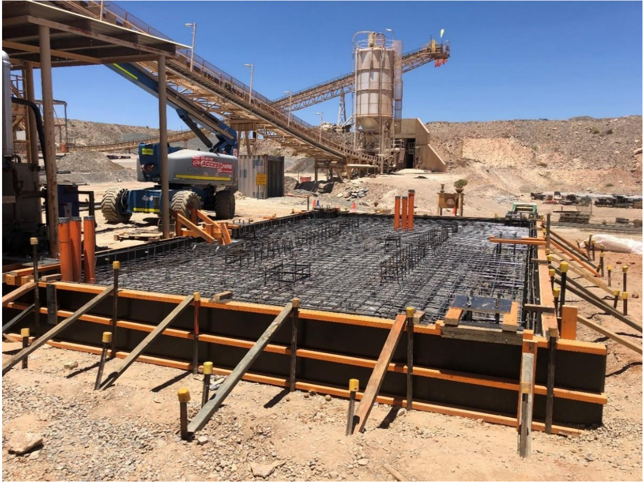
(Figure 4: Foundation for the new Acacia reactor unit being prepared for first concrete pour – view facing south.)
