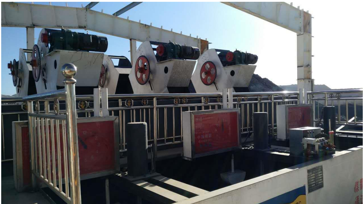
Figure 17-4: Installed Movable Screen Jigs of the Wet Washing Plant
