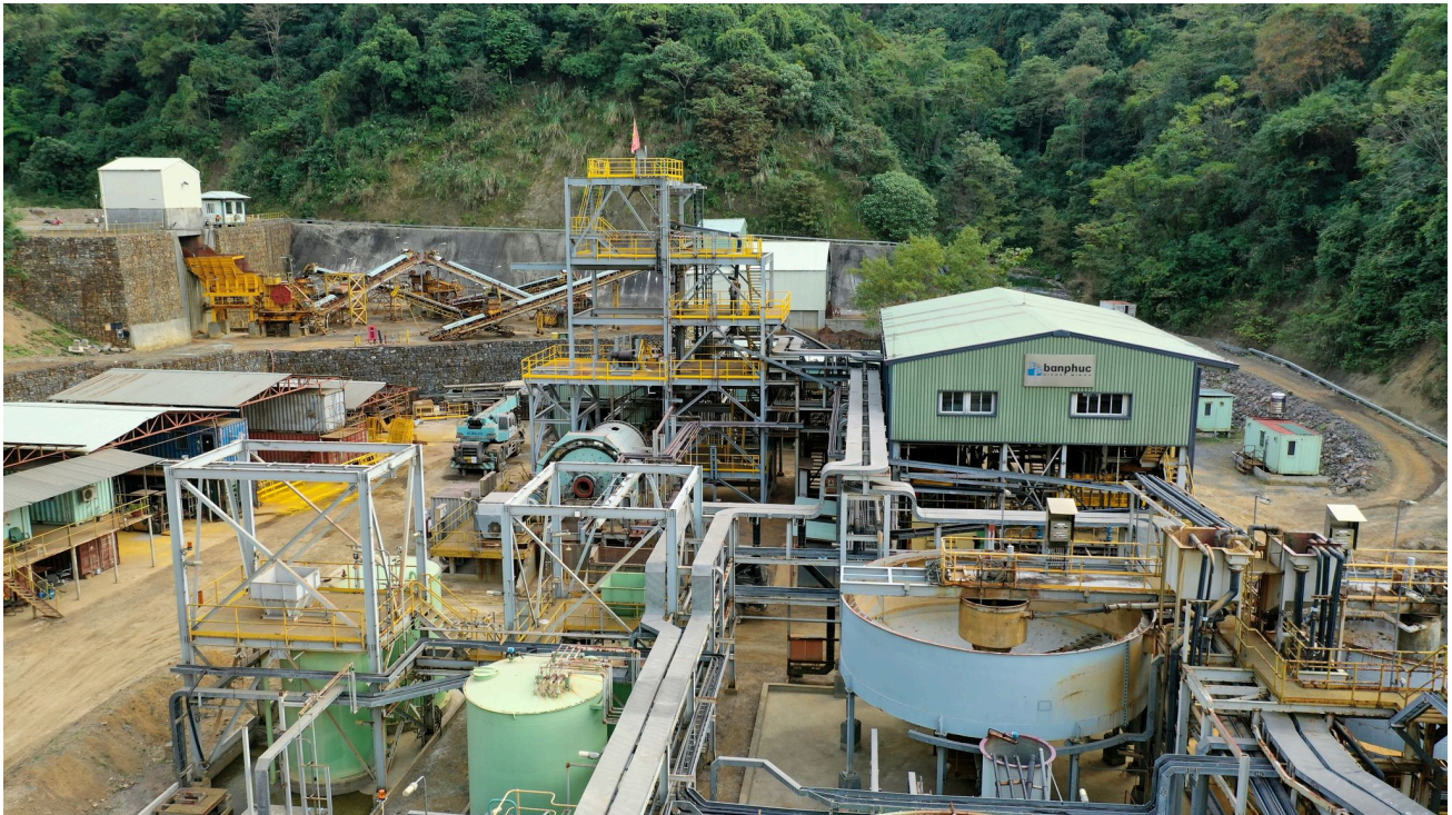
Figure 22 - Ta Khoa Processing Plant - existing 450ktpa Concentrator
