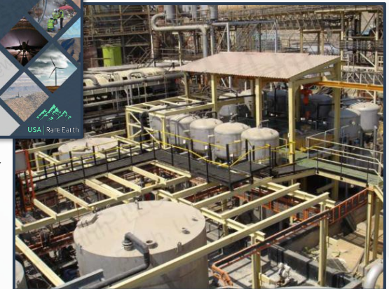
Industrial Scale CIX Plant installation Puritech IONEX System - Mine Site (Zambia)
